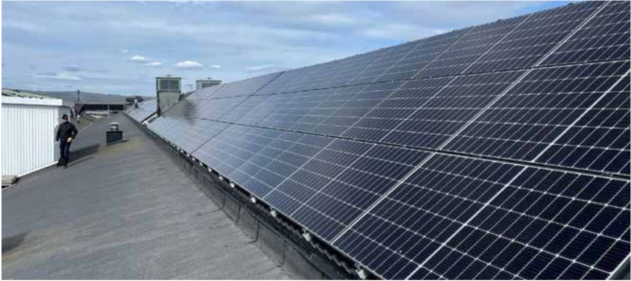
Örnsköldsvik's Largest photovoltaic power plant was installed in Hägglundsområdet in Gullänget. An investment of more than 4.5 MSEK. The maximum effect is 499kwp and is estimated to produce 415Mwh annually, which in turn reduces the climate impact by 195 tonnes of carbon dioxide per year.
